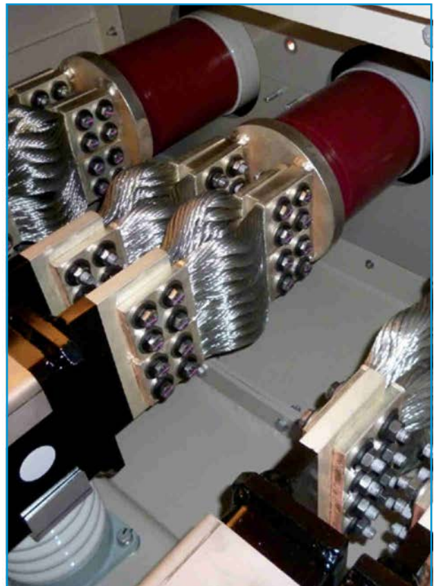
5000A generator connection
