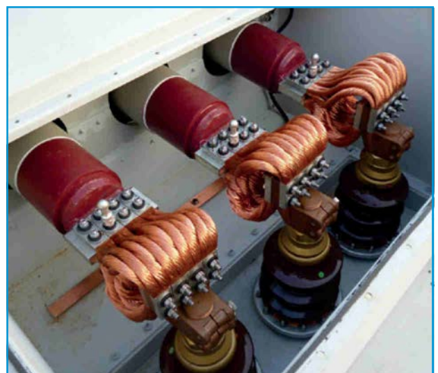
Copper braids to transformer
