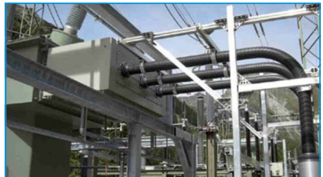
Switzerland - KW Löbbia: 17,5kV - 4000A
