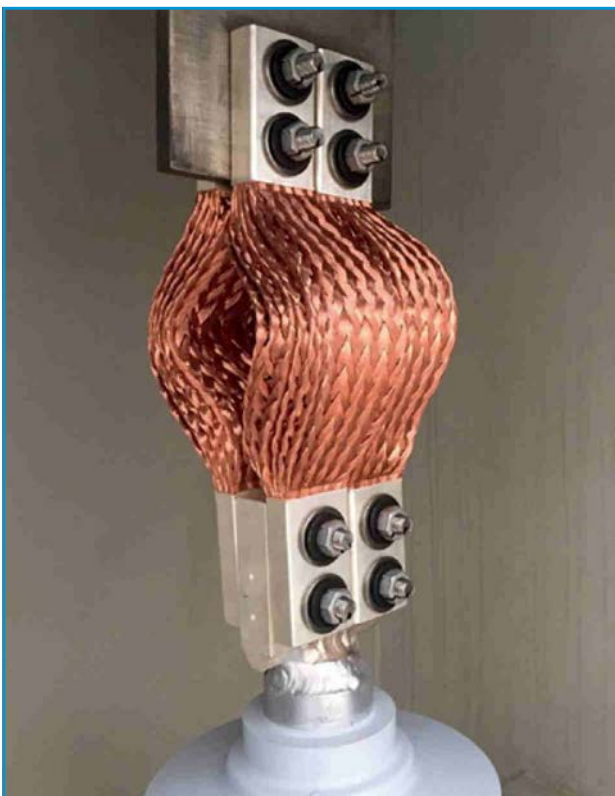
Copper braids to transformer
